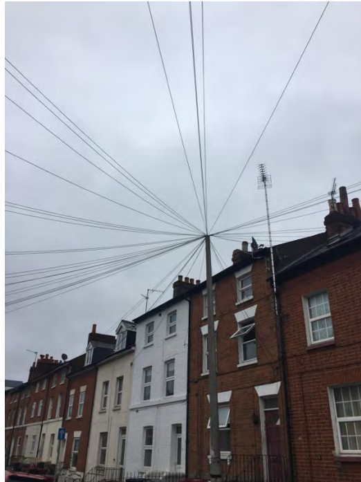
Figure 5.5.2 Overhead wires on a street with numerous HMOs.
